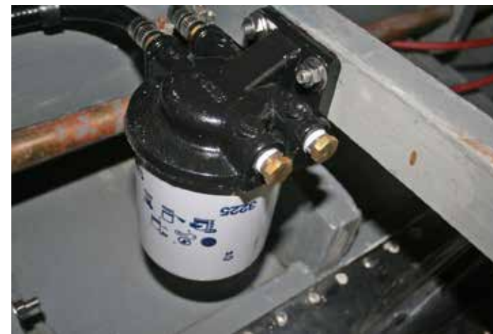
Fig 2 – Remote Gasoline filter -water separator
